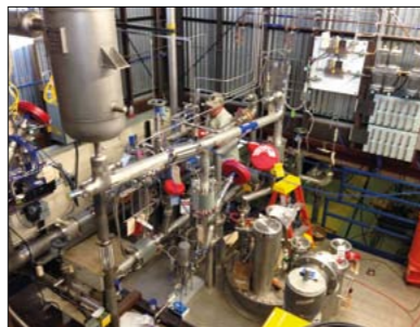
Fermilab technician John Najdzion, standing on top of the LBNE 35-tonne prototype cryostat, works on the piping for the cryogenic systems. (Image credit: Fermilab Media Services.)
